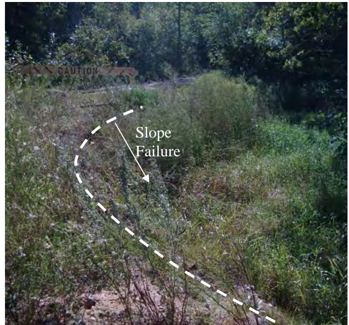
Figure 2.10 Slope Stability Issues off Gibson Drive August 2013
